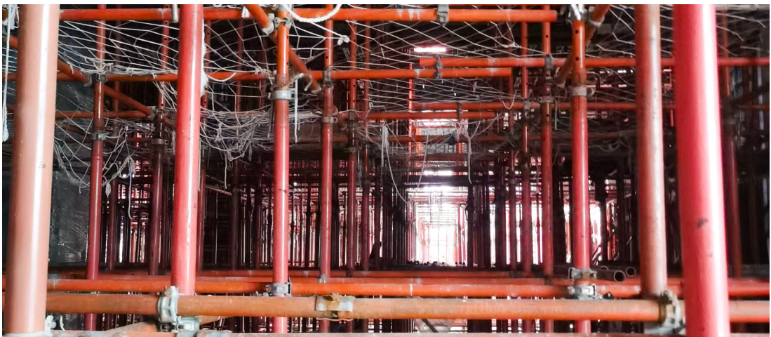
Construction Method of Independent Support and Aluminium Formwork 独立支撑 + 铝模施工工艺
