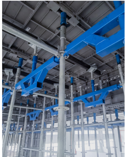
Reinforcement Scheme for Slab Panel with Heavy Loads 大荷载顶板加强方案
